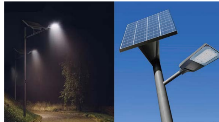
We can look at options to provide solar powered lighting along the footpath
